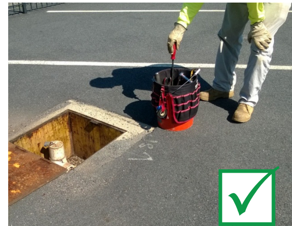
Hand tools stored off the ground in a designated container, out of the immediate work area
